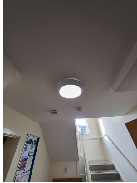
Lighting (Standard and Emergency Lights)
